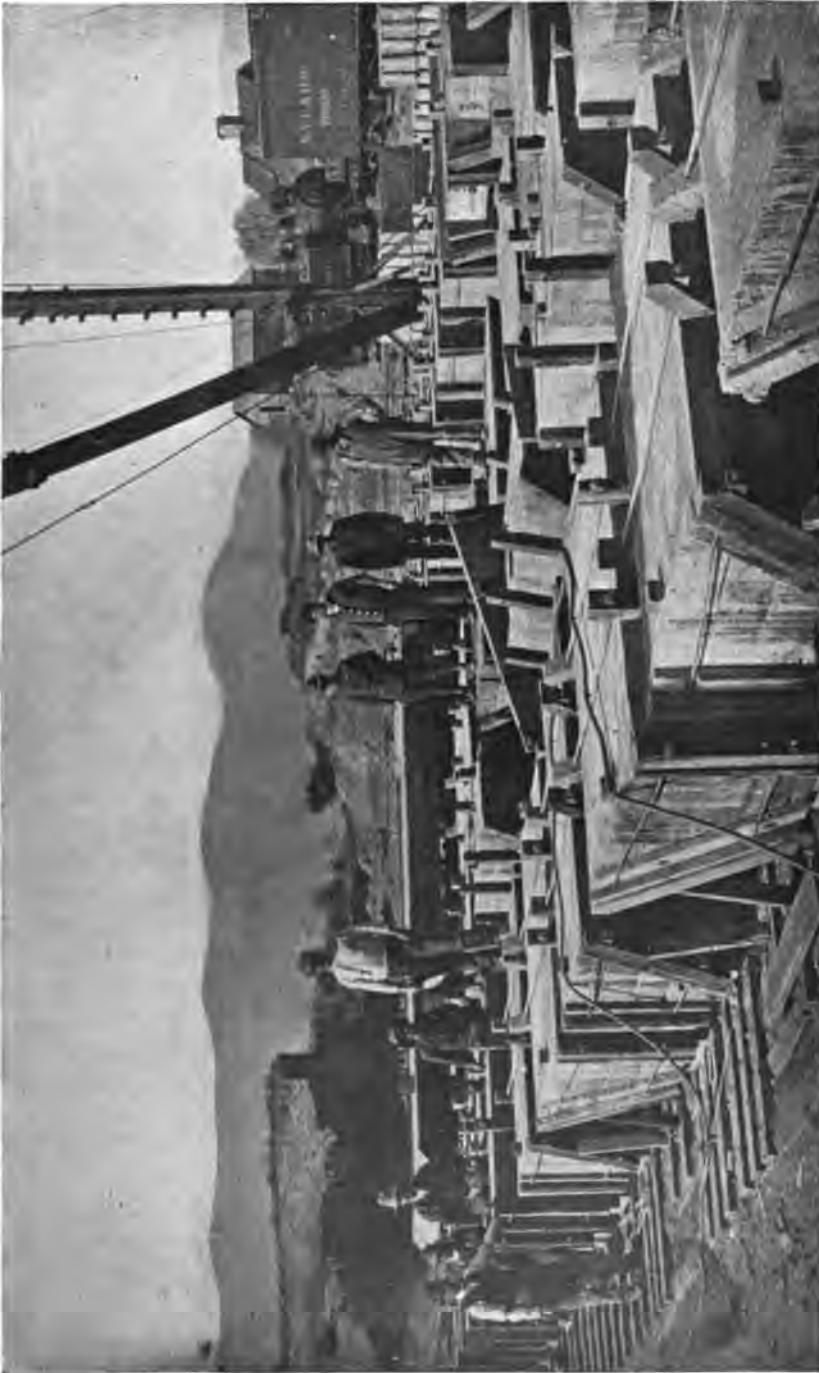
PLATE 39. —View of Blockyard at Olive Bridge Dam, Showing Forms and Derrick for Handling Blocks; also Traveler from which Forms were Filled.
